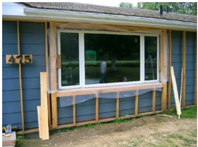
Figure 2. A photo by the author of his own house retrofit showing both the exterior wall being framed in and a new superinsulated window being installed in the rough opening of the old wall. Both of these are examples of how to retrofit both windows and walls with more insulation and a better performance window. The superwindow is described in the Fall 2005 issue of the Alaska Building Science News . It is a fiberglass framed quad-pane, krypton-fill window, 10 feet wide and 5 feet high with a measured R-value at approximately -20°F of 13.25 over a 36-hour period.
