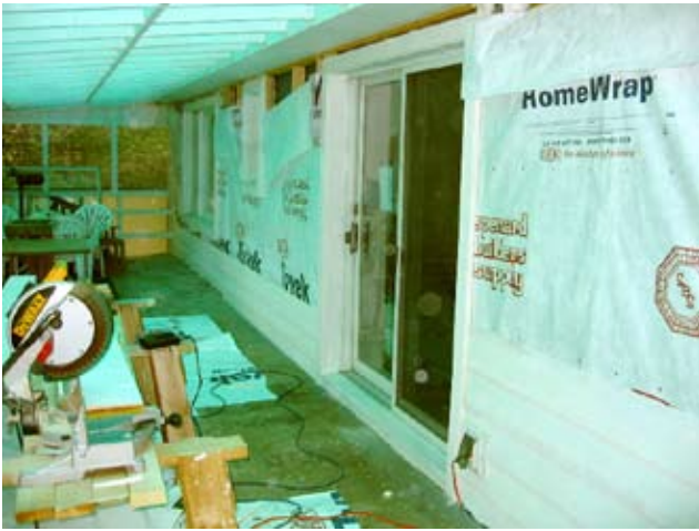
Figure 3. Shows another detail of the author's home in the final retrofit stages. The wall is being covered on the exterior with Tyvek® homewrap and the siding then installed such that cellulose insulation can be sprayed in the wall cavities and below the windows as the siding is attached. The finished wall is then sealed and the insulation is contained by the Tyvek® on the exterior. This system worked extremely well but it only worked well because the new window openings were sealed with foam sealant and the vapor barrier caulked to the inside of the window frame. The vapor barrier itself was of good quality, and had the confidence of the retrofit team that it did indeed stop most of the moisture at the inside wall. These two photographs (Figures 2 and 3) are indications of one way to amply retrofit a wall of a house to achieve a good result. The wall shown in Figure 3 resulted in approximately an R-27 wall when it was originally about R-11. This nearly tripled the insulating value of the wall.
