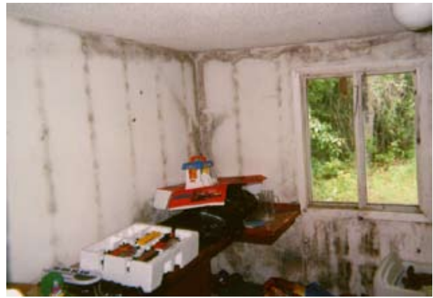
Figure 1. This photo shows several aspects of a house, which is poorly insulated at the studs such that you see condensation and mold not only at the top of the wall where the wall plate is, but also in the corner and at each stud. This is an extreme example of a phenomenon called "ghosting of the studs" where the surface of the wall on the inside of the stud is cooler and therefore condenses out moisture and other vapors on the cool surface first. In the case shown, the problem is fairly horrible with the resulting mold on every cool surface of the inside of the building. Retrofit would solve this by insulating on the exterior or the interior and using good vapor barrier sealing to keep moisture from getting to cold surfaces. The existing condition may also be a result of a fairly tight air seal causing exceedingly high relative humidity levels in the building. Photo by Scott Waterman.
